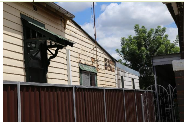
Detail of acrylic paint peeling and timber rot on the north elevation.
