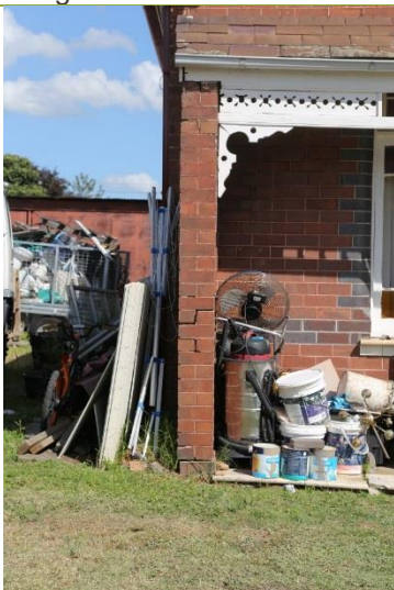
Detail of cracking in wall supporting verandah roof.
