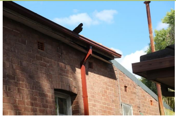
Detail of deteriorated eave on the north elevation.
