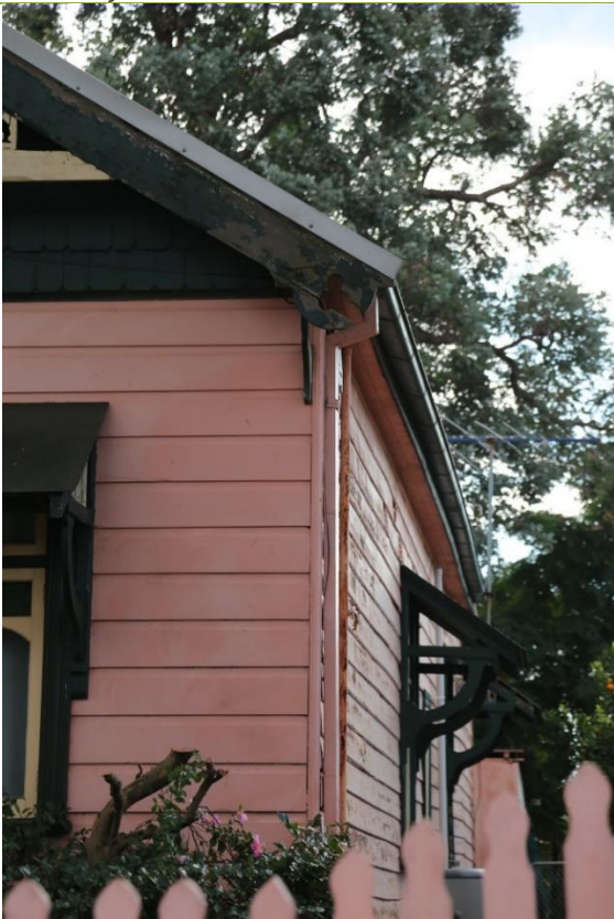
Detail of deteriorated timber to barge board.
