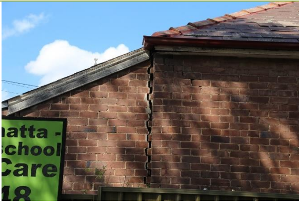
Detail of cracking in brickwork on the north elevation.
