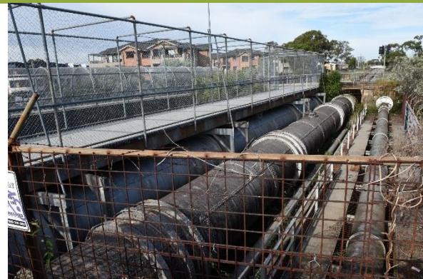
View of pipelines from Military Road, Guildford.
