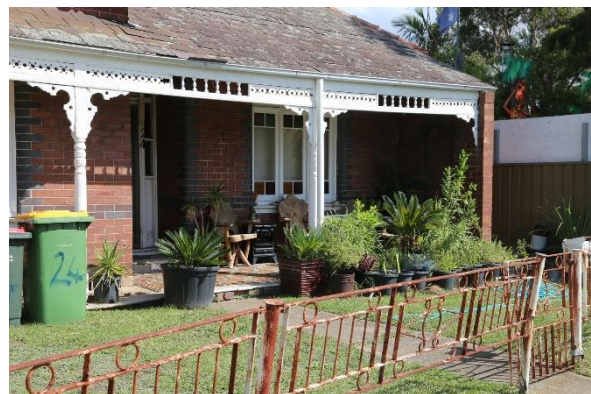
Detail of front façade and corroded fence.
